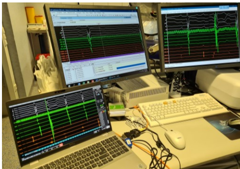
Parallel setup of displays next to each other; on the notebook screen the signals of EP-TRACER 2, on the 21" monitors the signals of the Labsystem Pro
